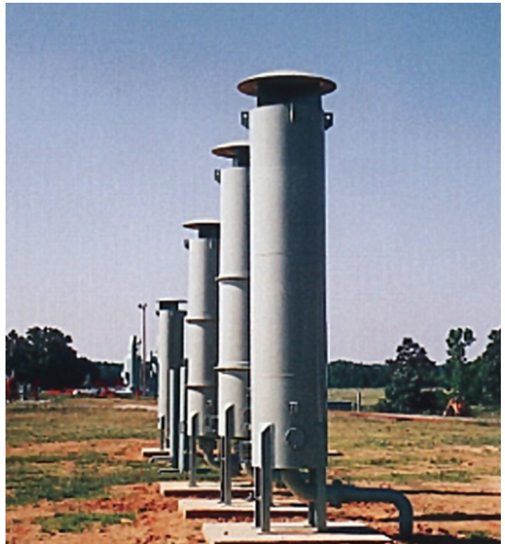
Multiple BDSS's (with optional weather hoods) serving numerous compressors.
